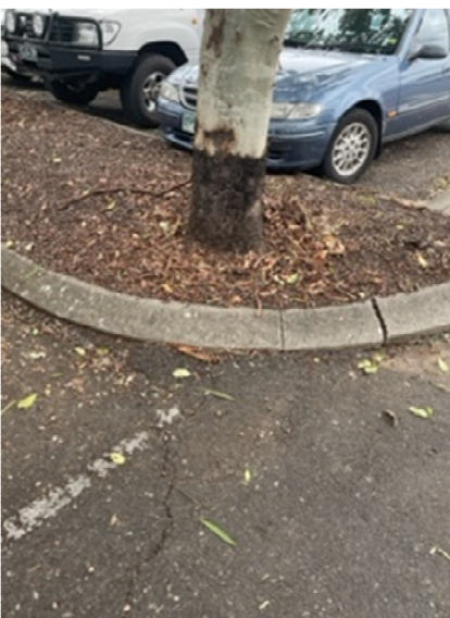
# 02. Showing root damage
