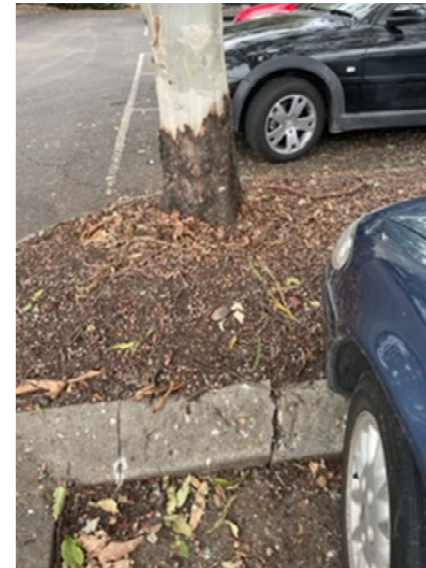
# 02. Showing root damage
