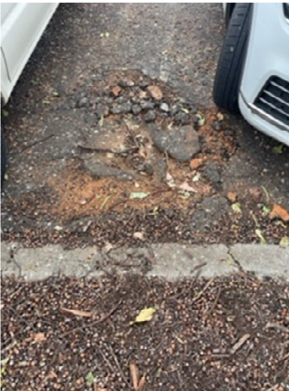
# 01. Showing root damage
