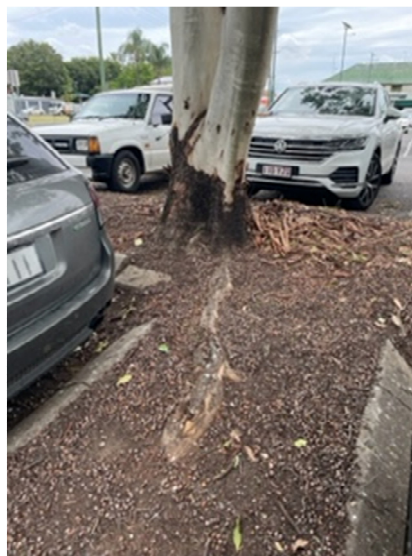
# 01. Showing root damage
