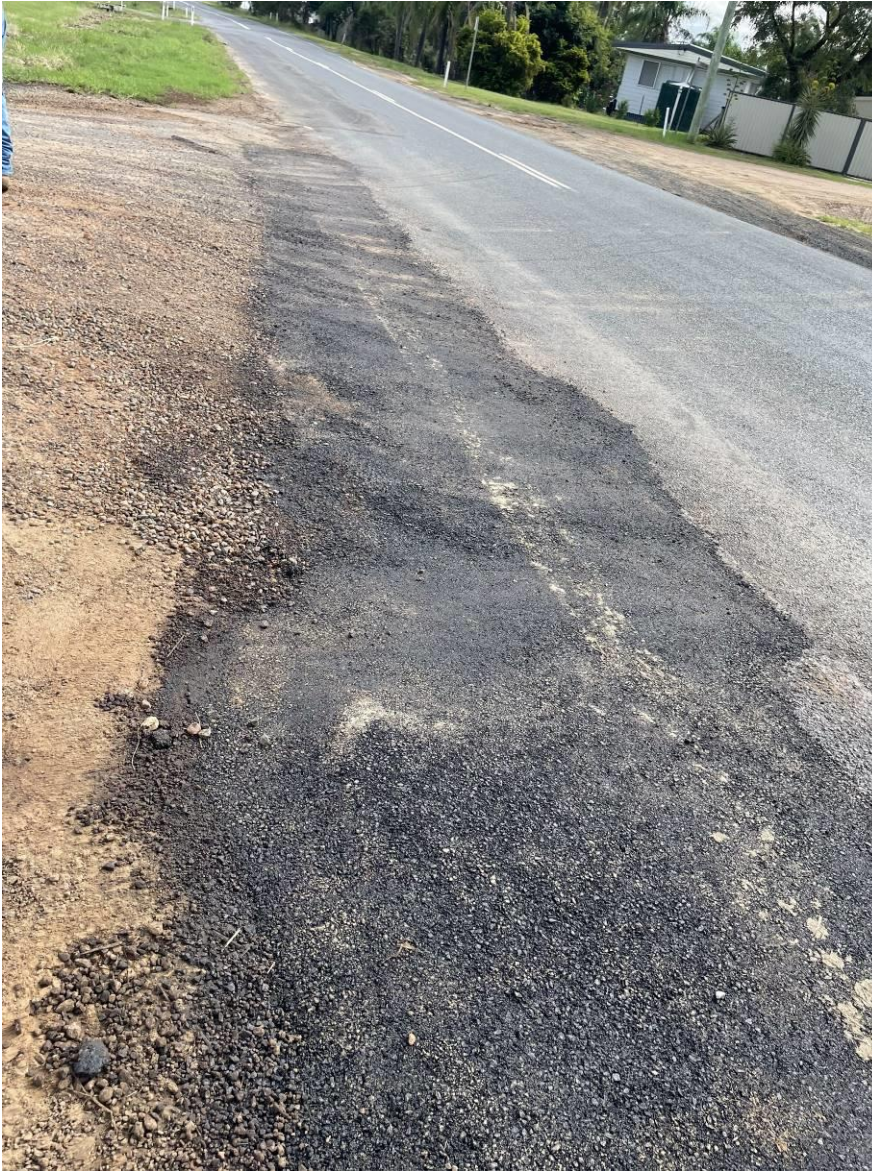
Figure 88 Entry has been patched.
