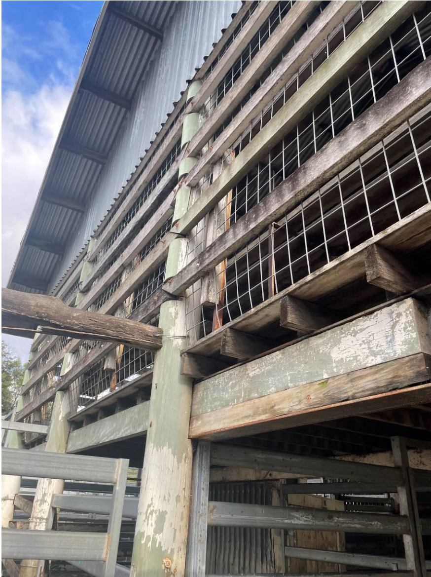
Figure 32 All seating is braced on the outer posts - not structurally sound
