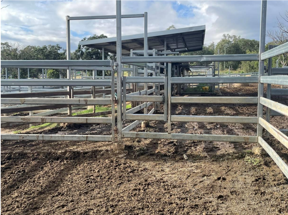
Figure 46 PA Gate in Vet Crush/Dip area. Top and bottom rails do not move. Serious Hazard.
