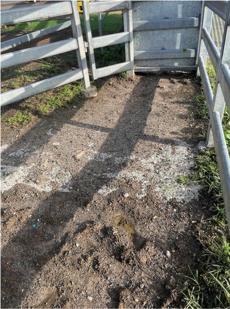
Figure 58 Loading Ramp surface not adequate. Concrete not adequately placed. Cattle and horses prefers steps not inclines.
