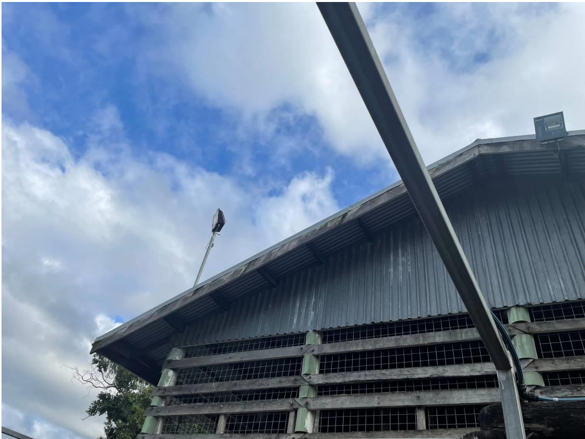
Figure 62 One Flood Light Point South East, One Flood Light Pointing East
