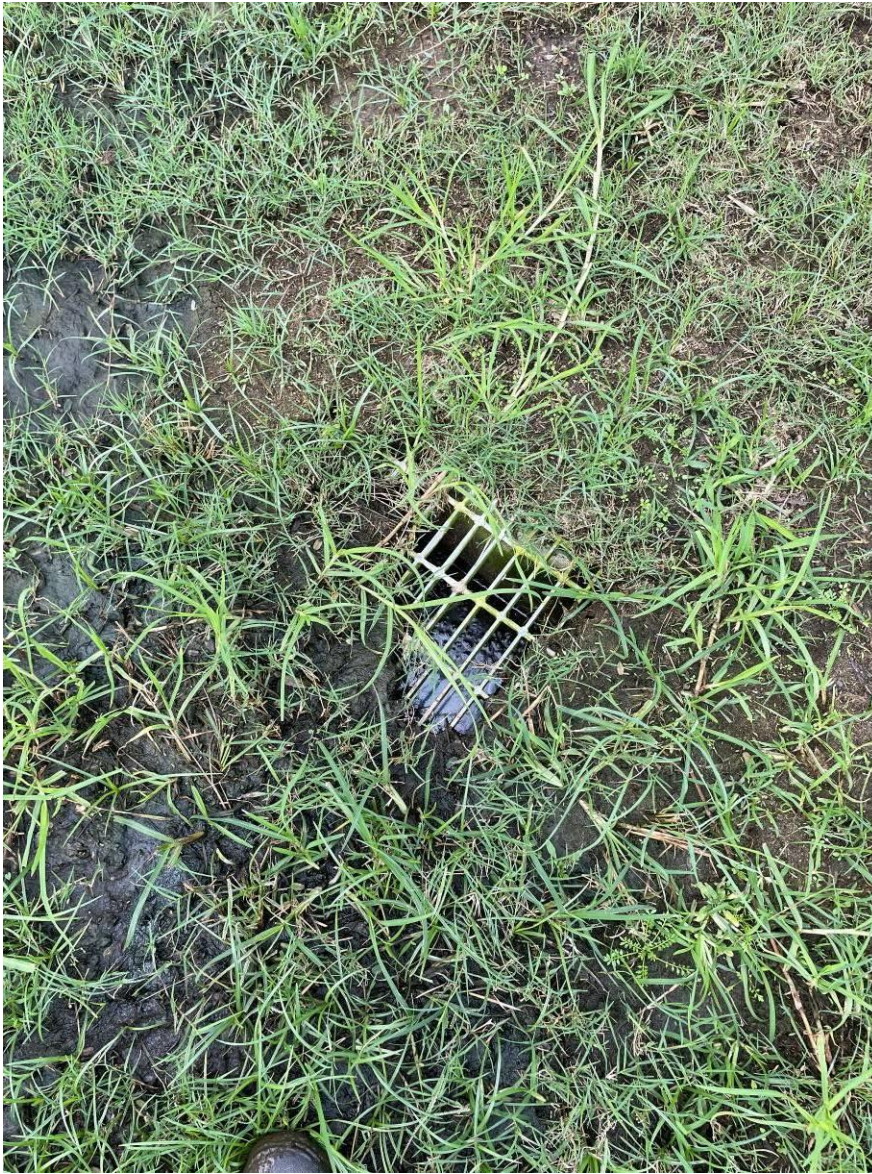
Figure 5 Stormwater Pit - located at Northern side of yards - filled with effluent.
