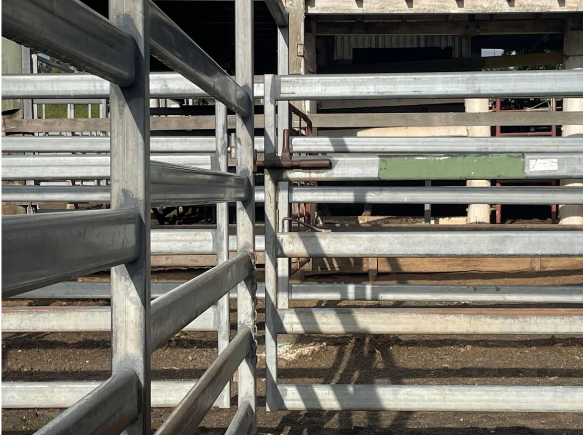
Figure 63 Gate locks installed upside down – multiple have.
