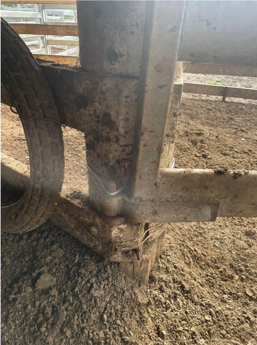
Figure 33 Makeshift used to hold gate into the pavilion in place.
