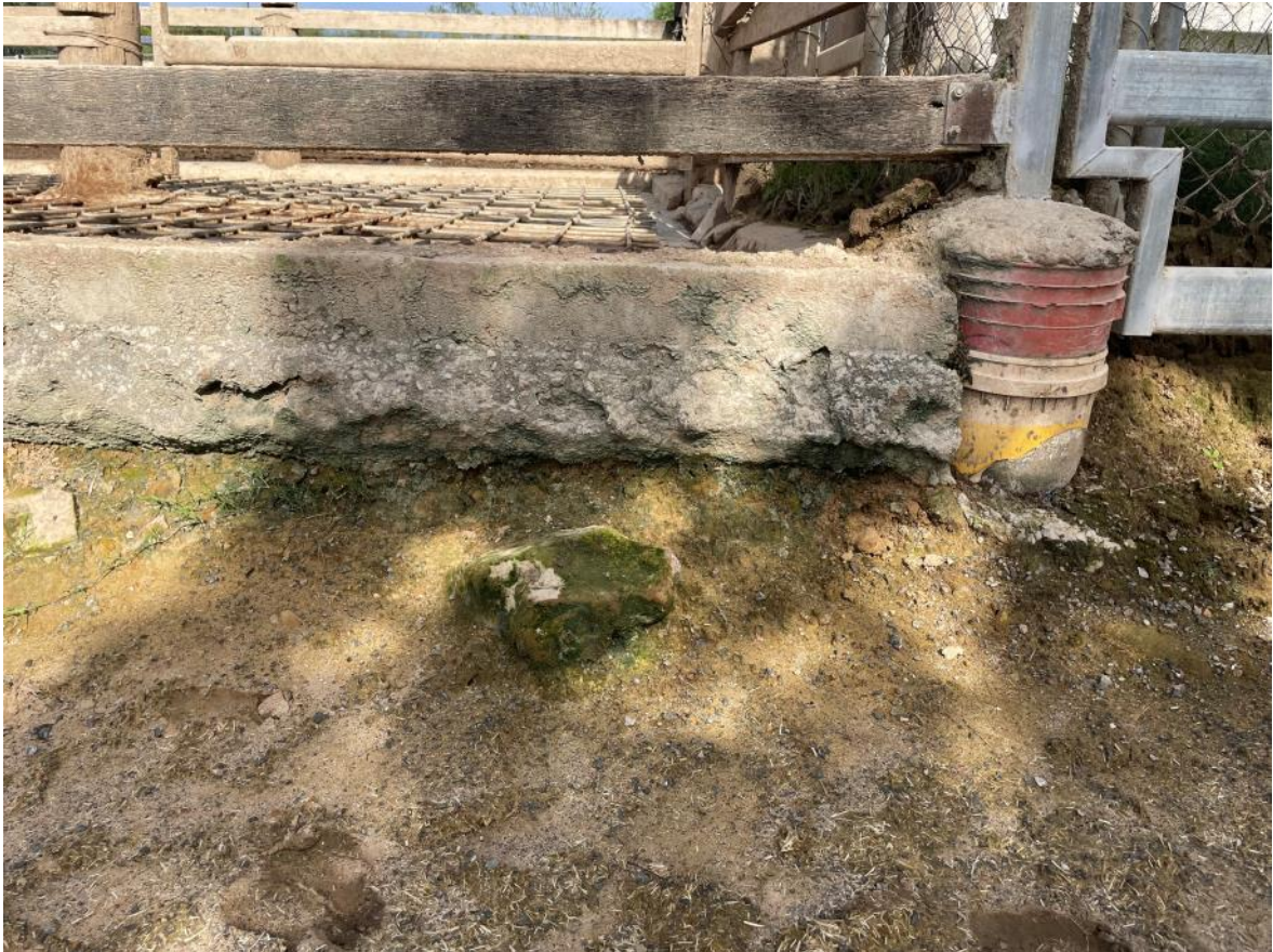
Figure 1 Leakage evident from Drainage Area at Rear of Dip – North Western Side.
