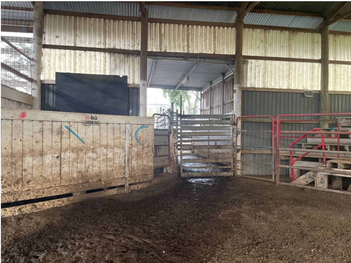
Figure 37 No Stormwater controls in place in the Pavilion.
