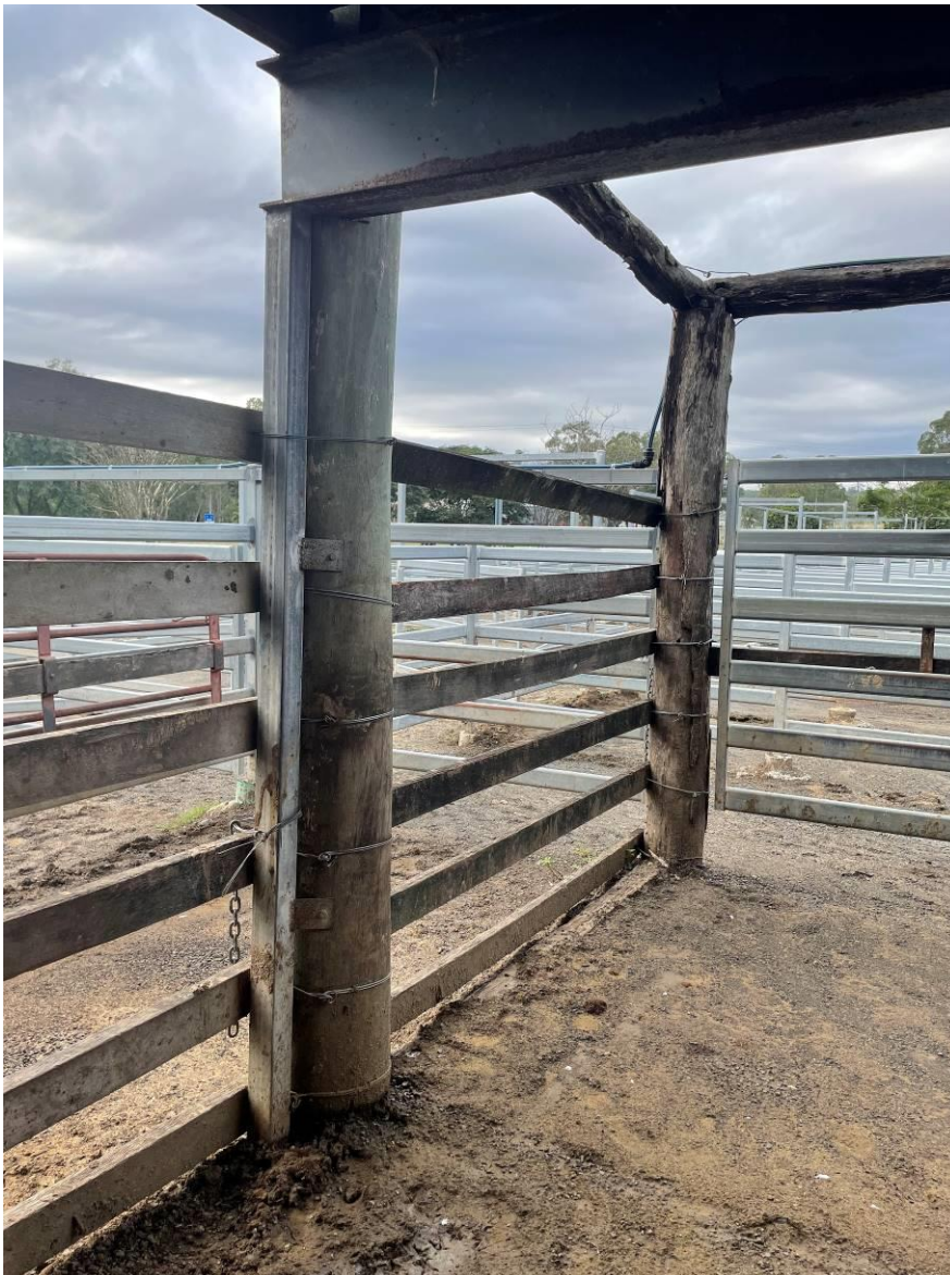
Figure 29 Steel post holding up bracing beam are inadequate.
