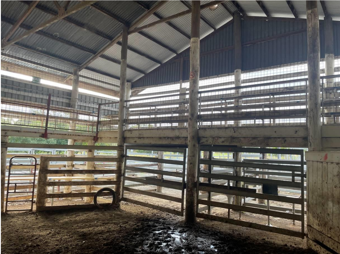
Figure 39 Seating is braced on back beams - not structurally sound
