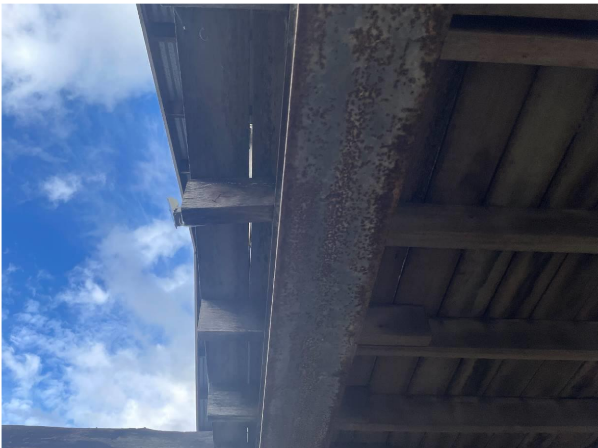
Figure 27 Supports on bracing beam are inadequate.
