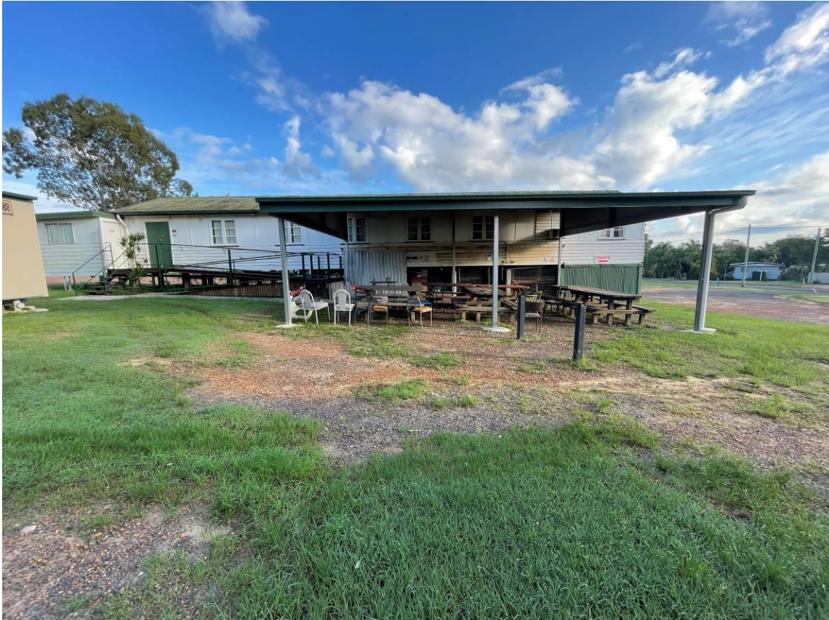
Figure 65 Lunchroom is not weather proof - floor floods.
