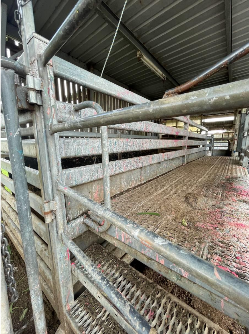
Figure 50 Platform access has trip hazards.
