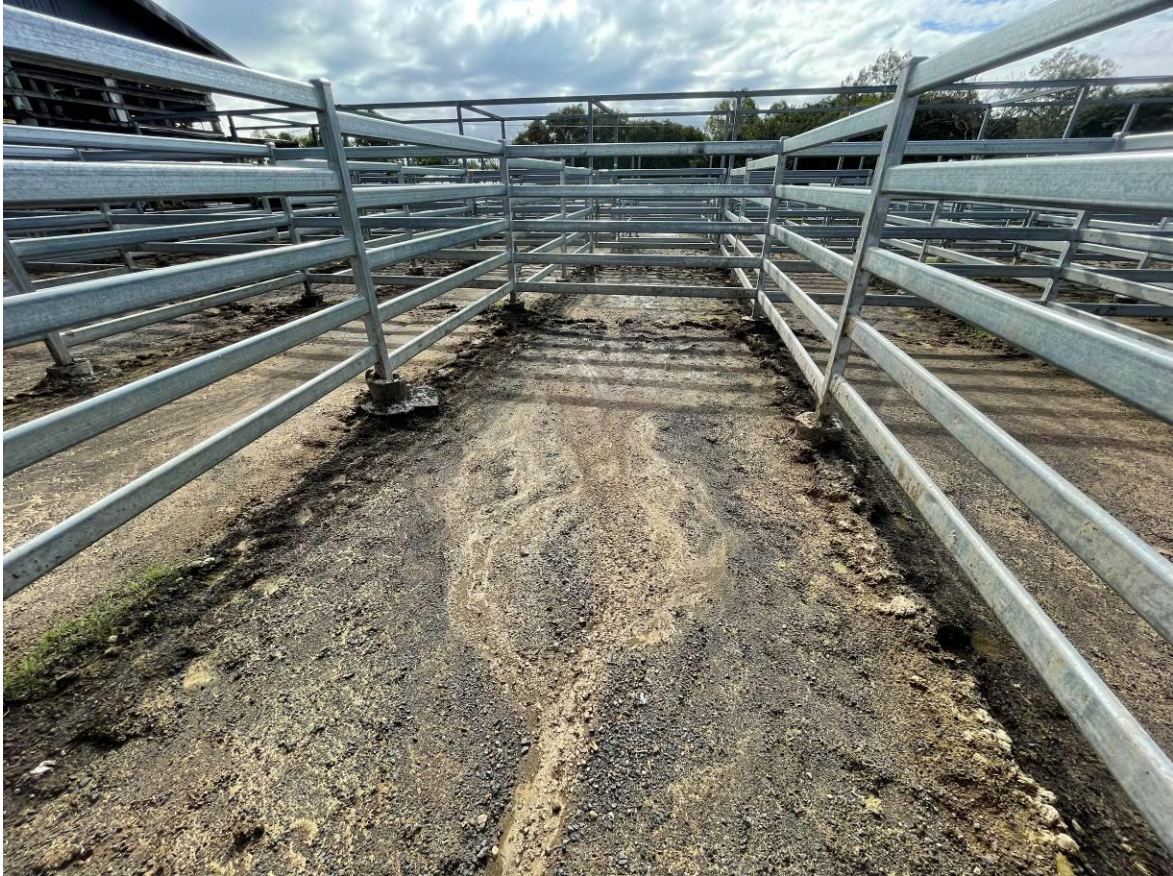
Figure 16 Yard surface is not maintained.
