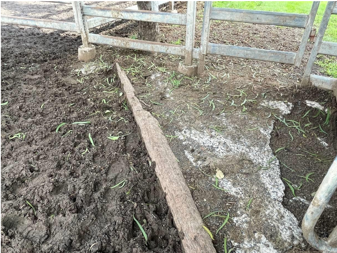
Figure 19 Broken Concrete on Entry/Exit Point. This is situated at the entry/exit to the Pond.
