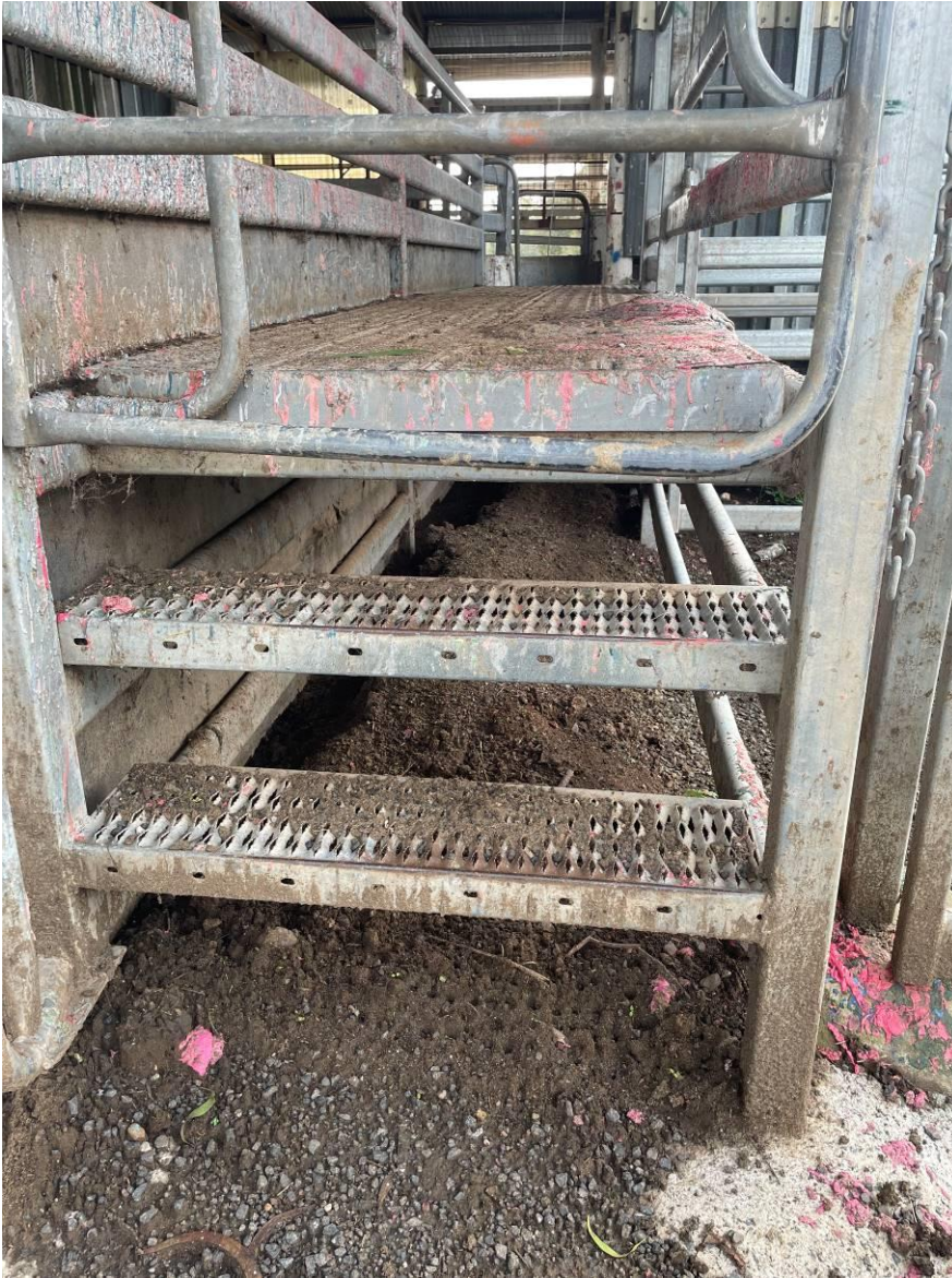
Figure 51 Steps on platform not compliant - no angle.
