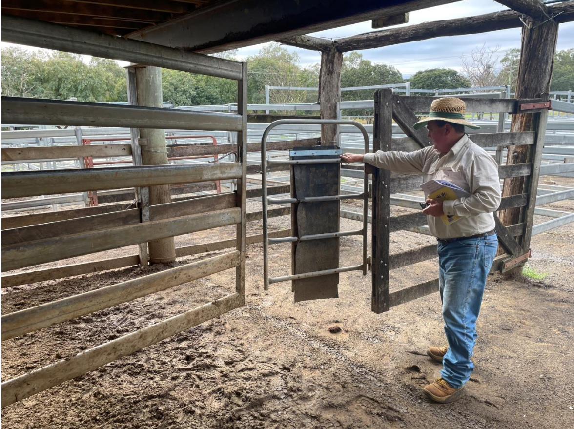
Figure 15 Gates into Pavilion used for Cattle - Serious Hazard
