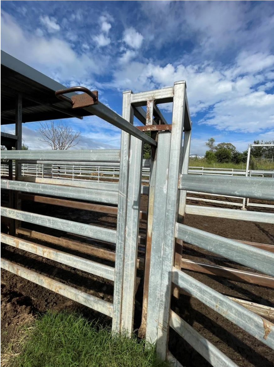
Figure 69 Hazard on entry gate to vet crush
