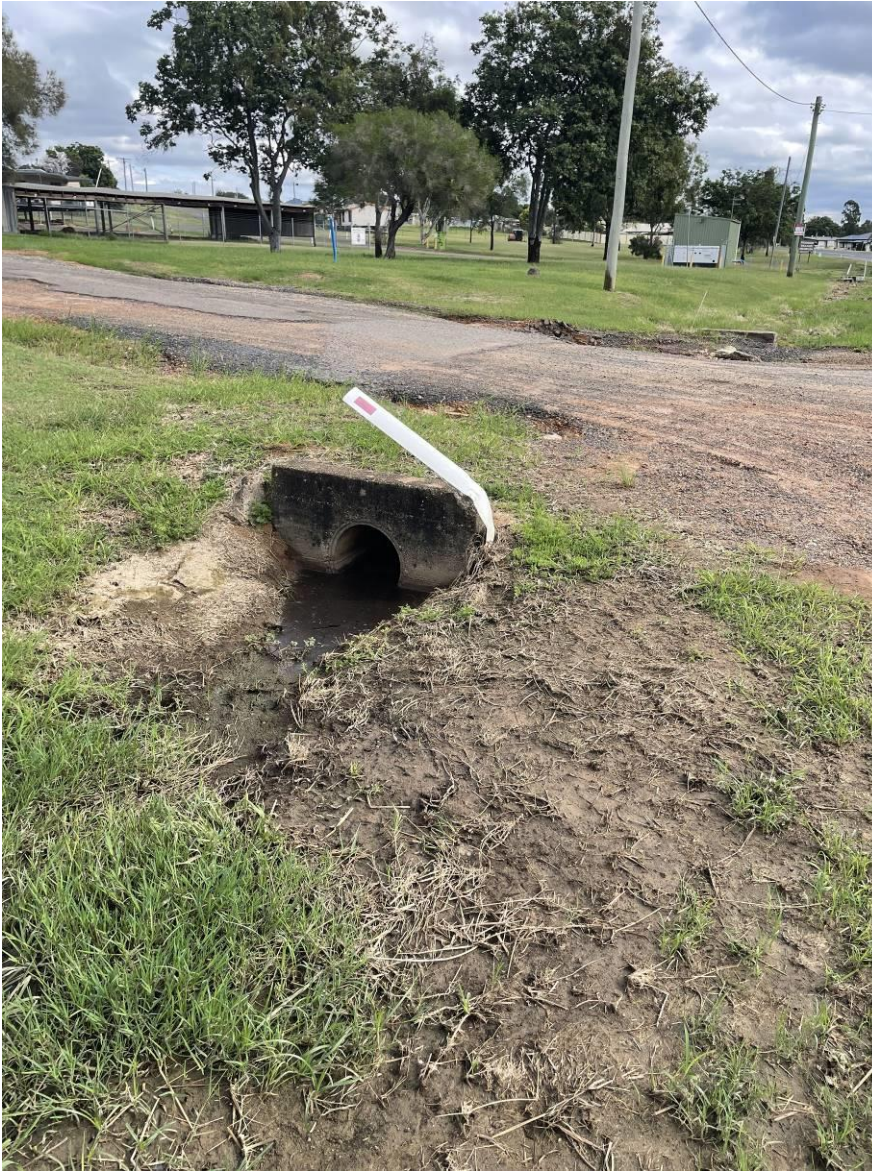
Figure 87 Damaged by vehicles.
