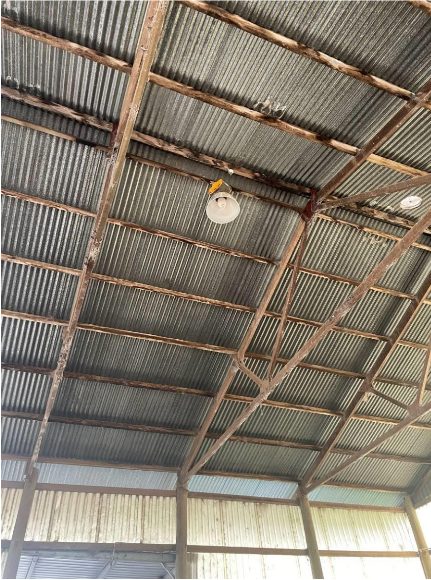
Figure 36 Lighting in the pavilion is inadequate.
