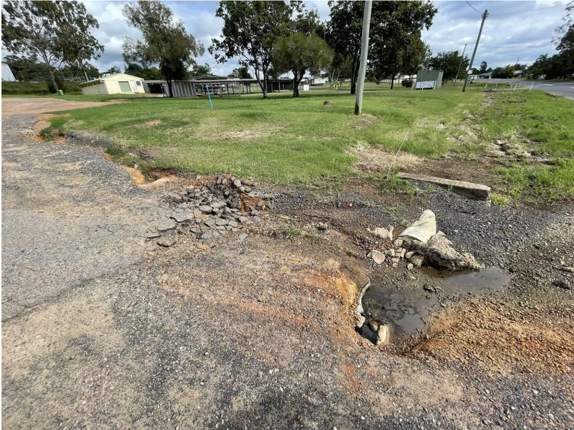
Figure 85 Driveway is eroding.
