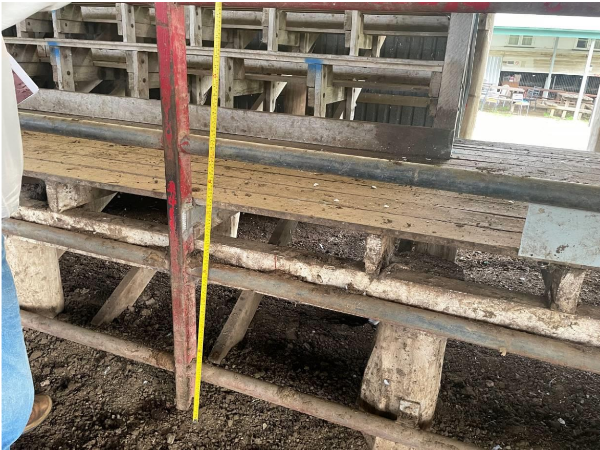
Figure 26 Gaps between too bars in fencing between animals and buyers are too wide inside Pavilion.
