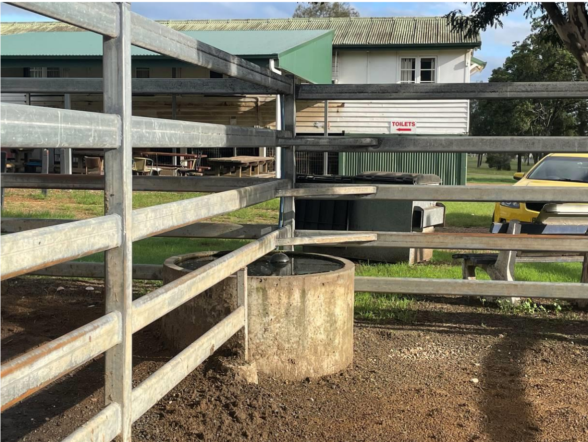
Figure 55 Water Trough mitigation not compliant.
