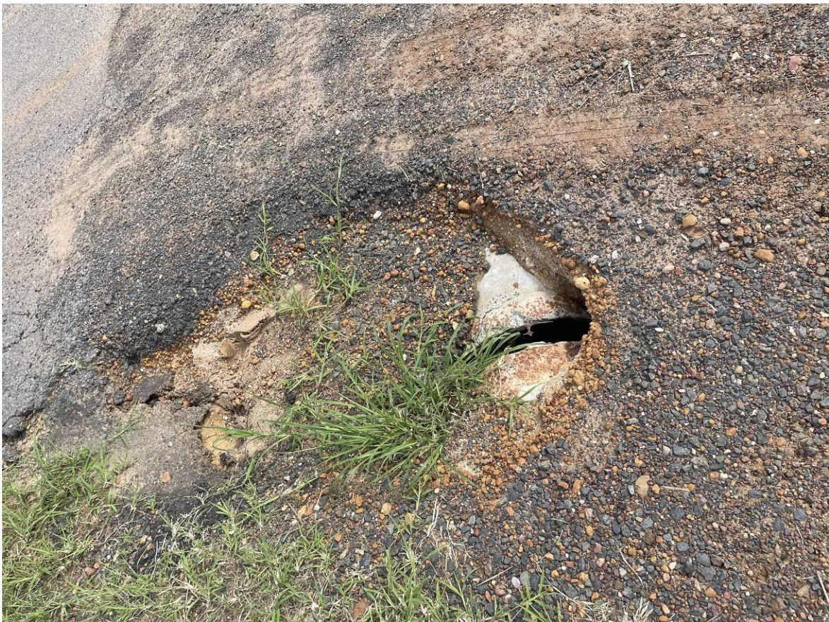
Figure 86 Pipe under driveway is broken – exposed through driveway.
