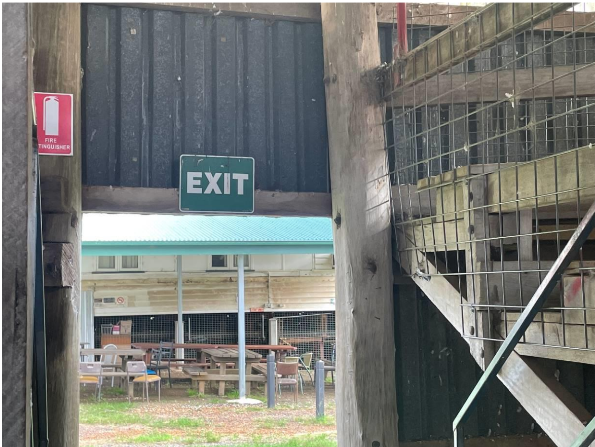
Figure 99 Fire Extinguisher and Exit Sign
