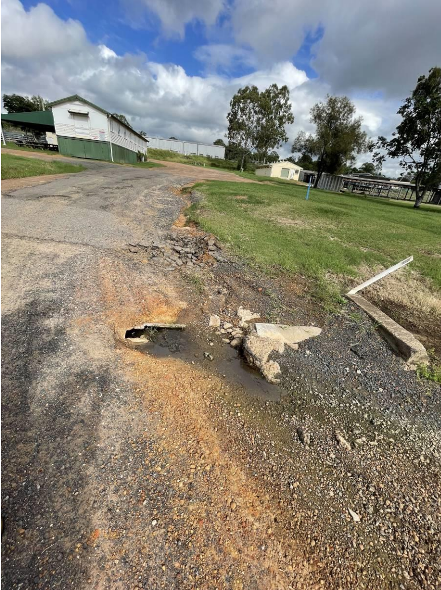
Figure 83 Under Driveway Pipe is broken.
