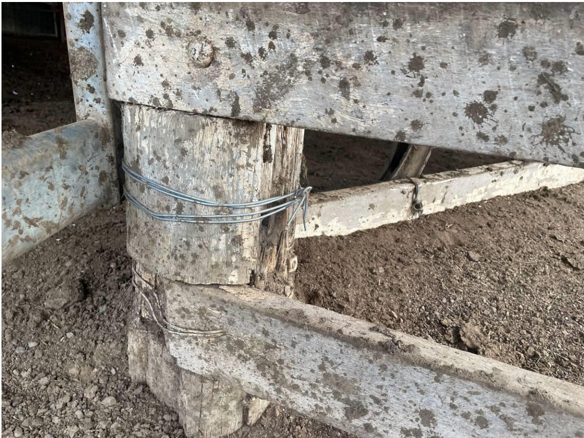
Figure 30 Makeshift tie holding on frequently used gate into the Pavilion.
