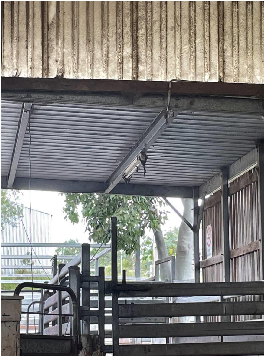
Figure 35 Lighting in the pavilion is inadequate.
