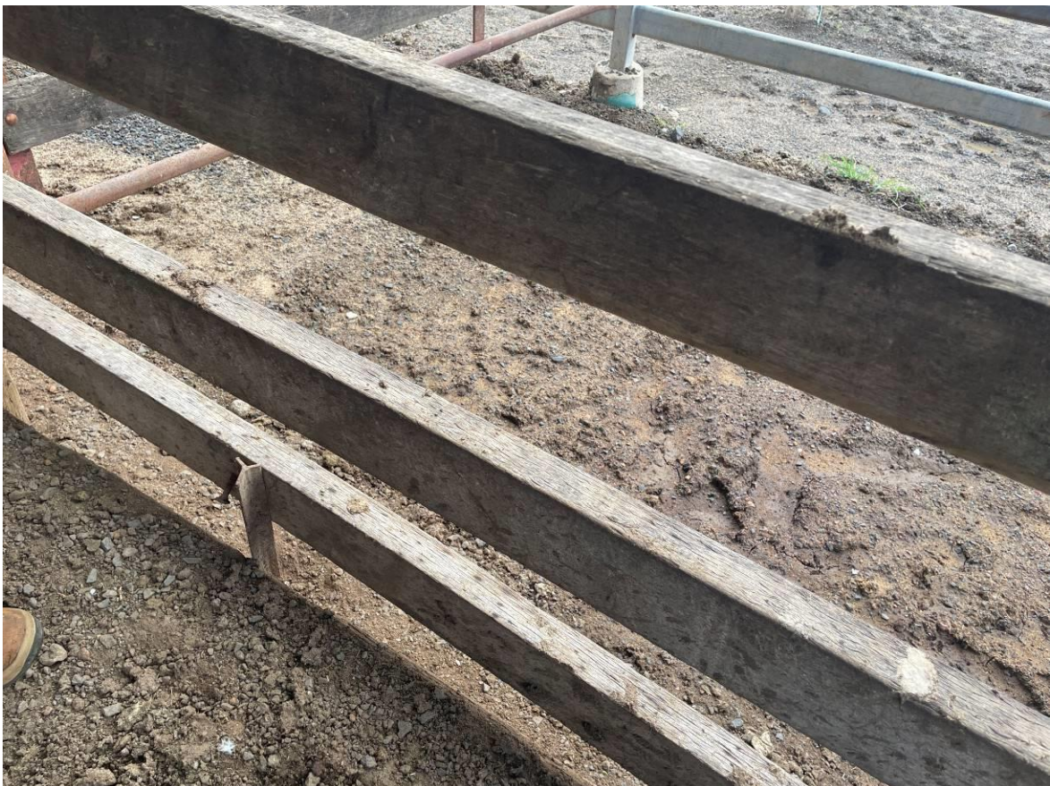
Figure 31 Star picket used to fix retaining wall - inadequate
