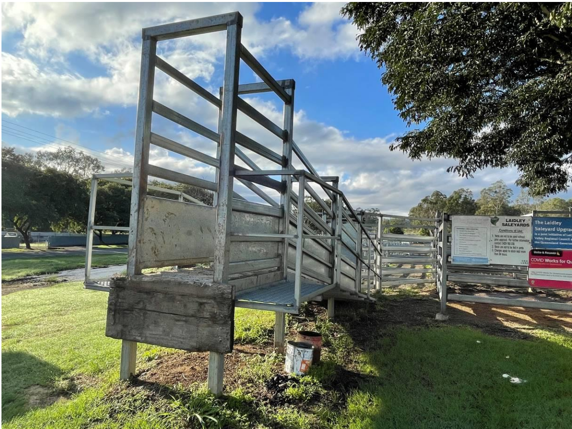
Figure 59 Loading Ramp (Northern Side) not compliant.
