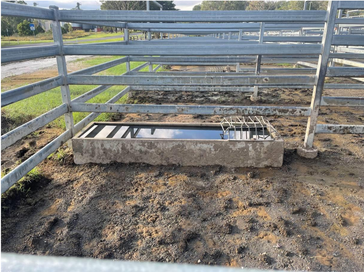
Figure 54 Water Trough with damage on north side of yards.
