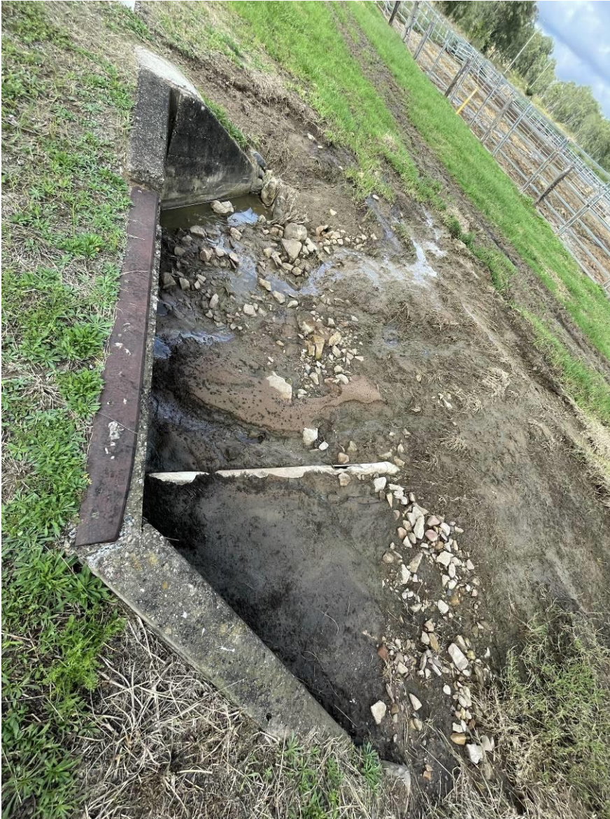
Figure 6 Stormwater Drain - pipe from stormwater pit broken.
