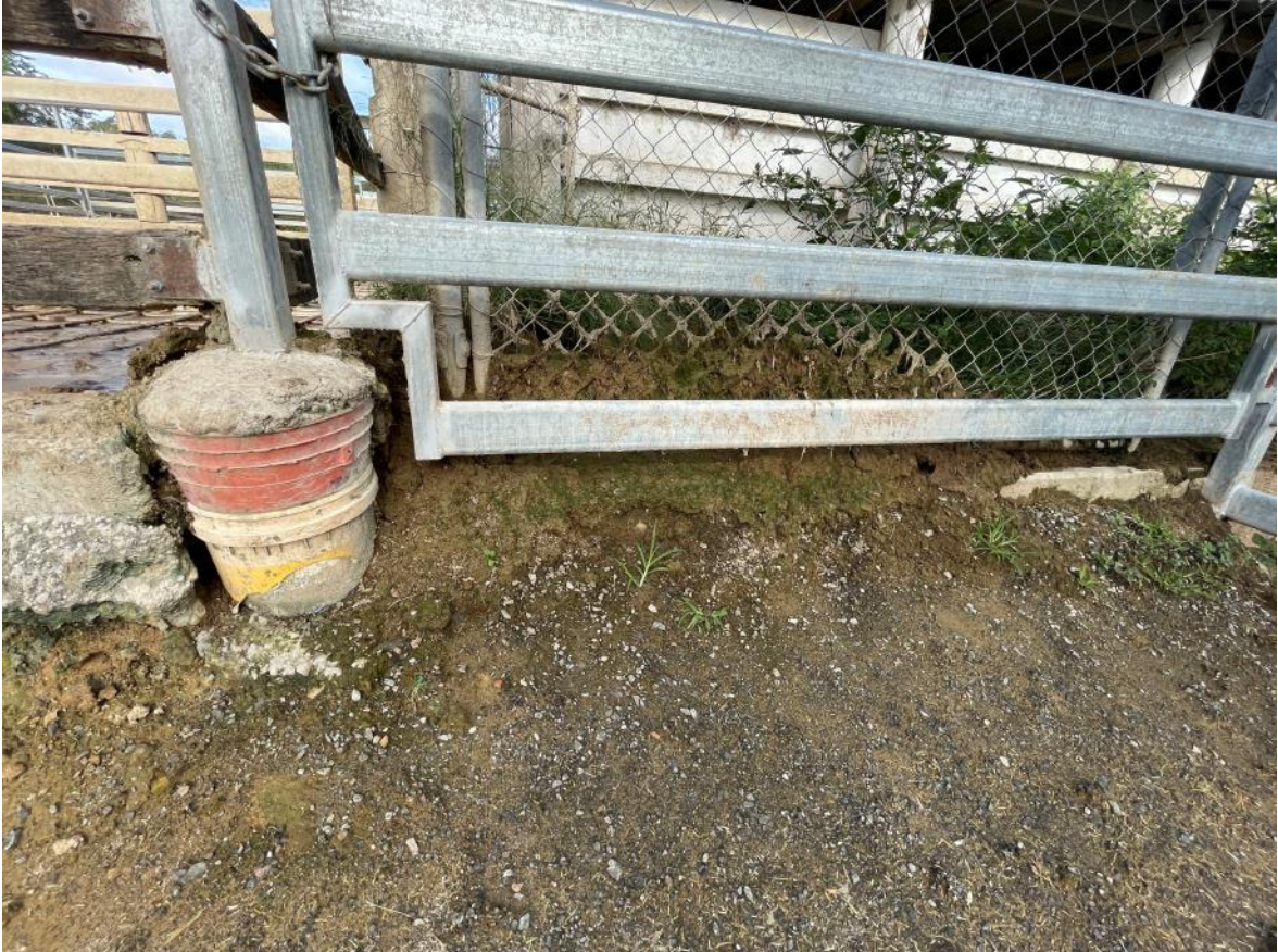
Figure 3 Runoff - Potential Leakage from Dip – Overflow noted from build up on the fence surrounding the Dip
