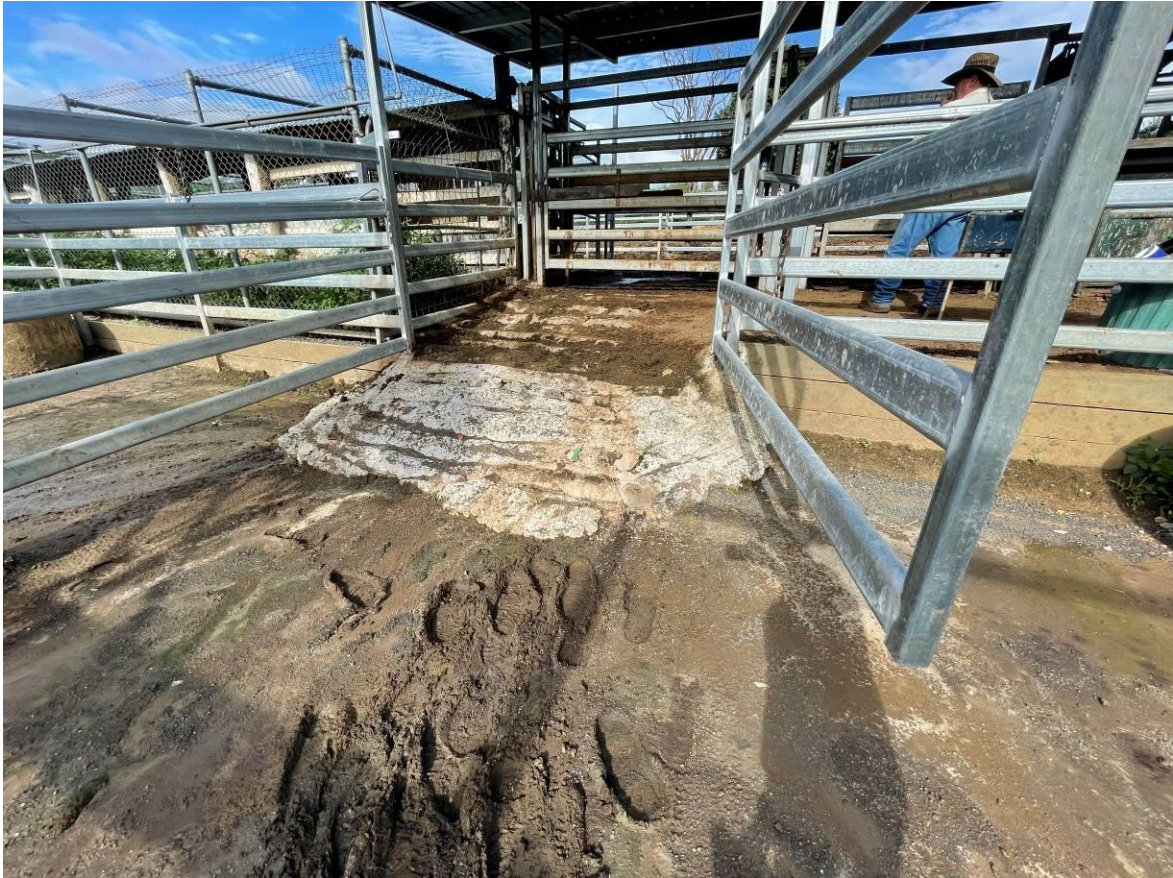
Figure 67 Ramp not compliant from crush
