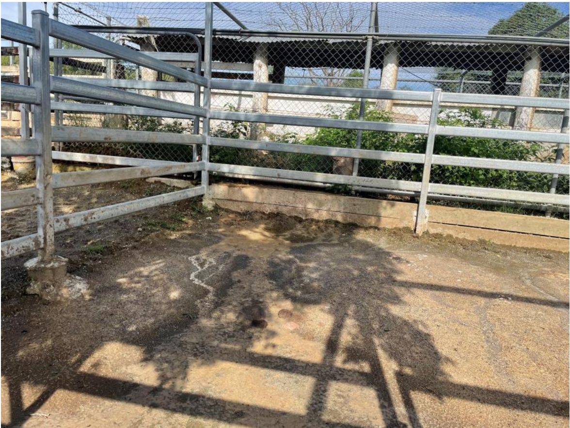
Figure 2 Runoff - Potential Leakage from Dip. Coming from Retainer wall and leaking through.
