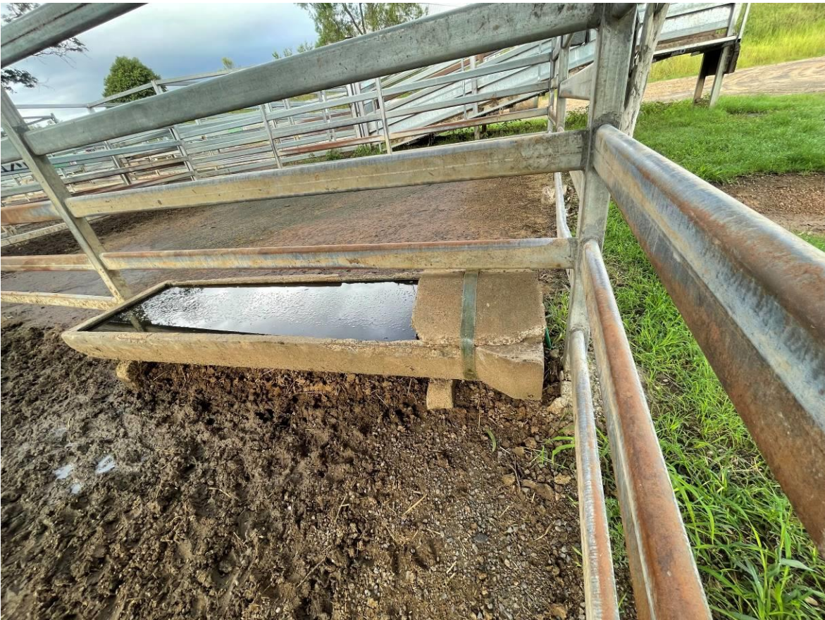
Figure 56 Water Trough damaged south western side of the yards.
