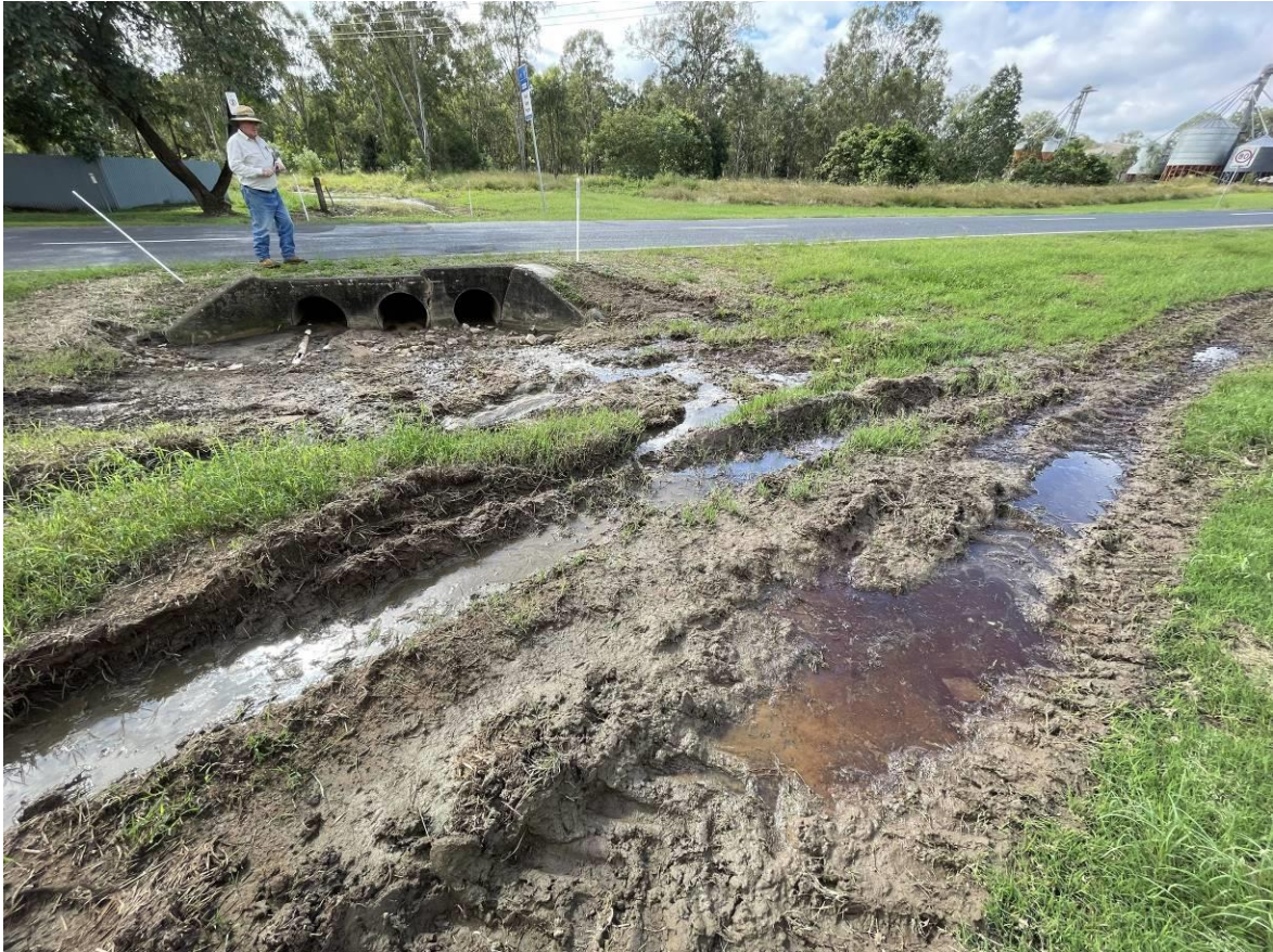
Figure 10 Effluent Flowing into Stormwater Drain which runs under the Laidley Rosewood Road
