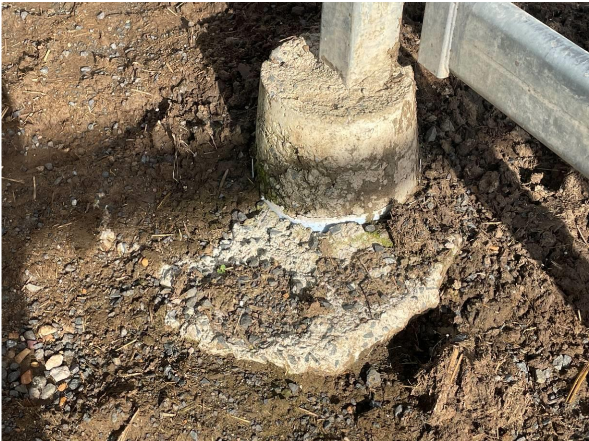
Figure 74 Footings on posts cracking
