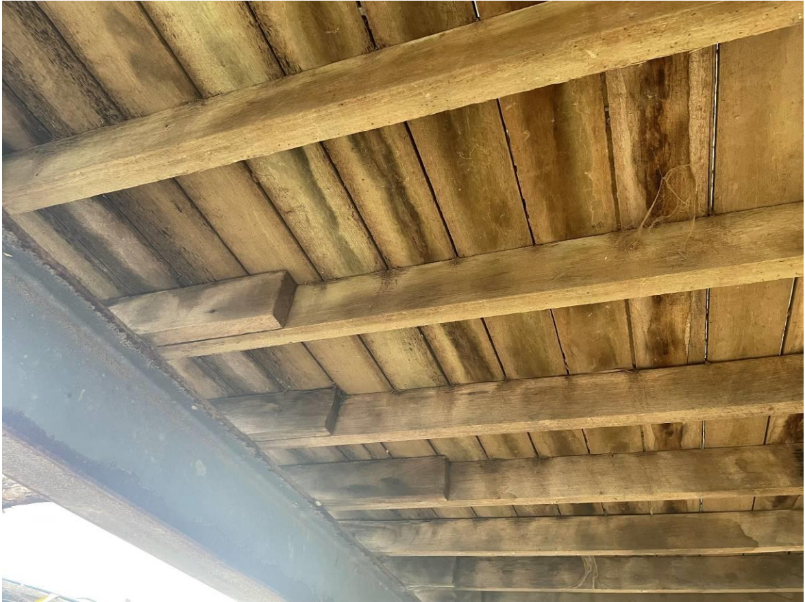
Figure 28 Supports on bracing beam are inadequate.
